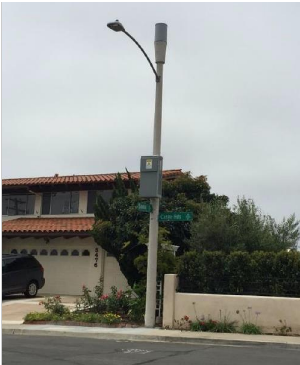
Figure 1: Antenna concealed within a single shroud (or radome) with a tapered cable shroud between the antenna and pole-top
