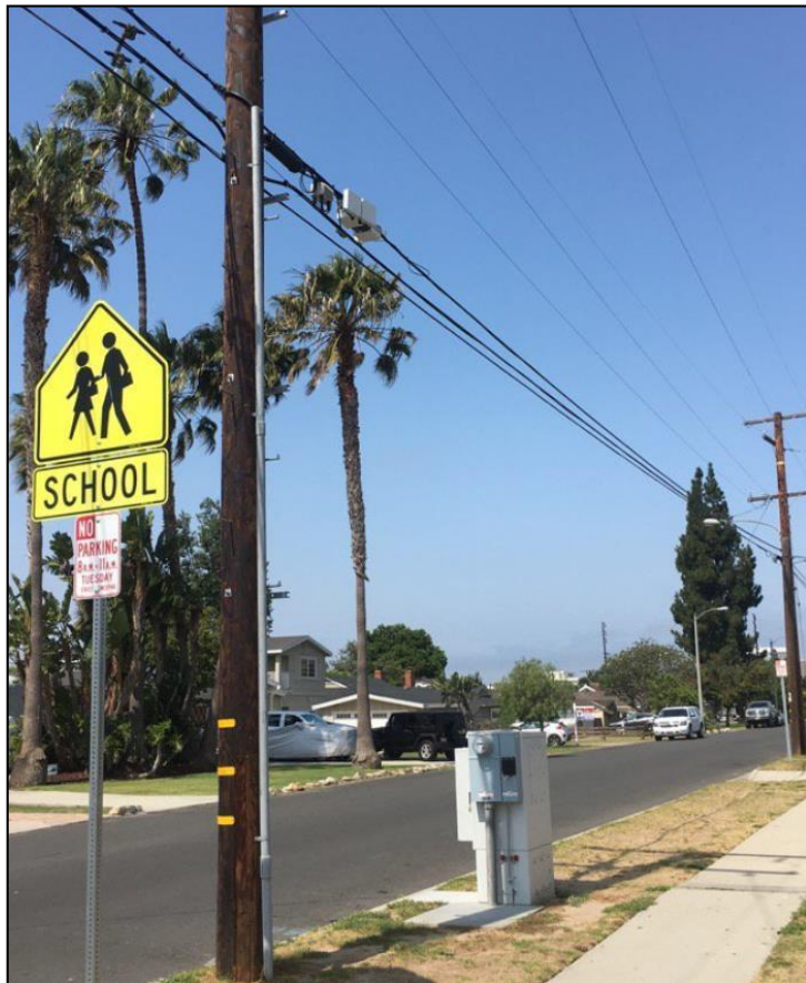
Figure 8: Strand-mounted wireless facility with a ground-mounted remote power source.
