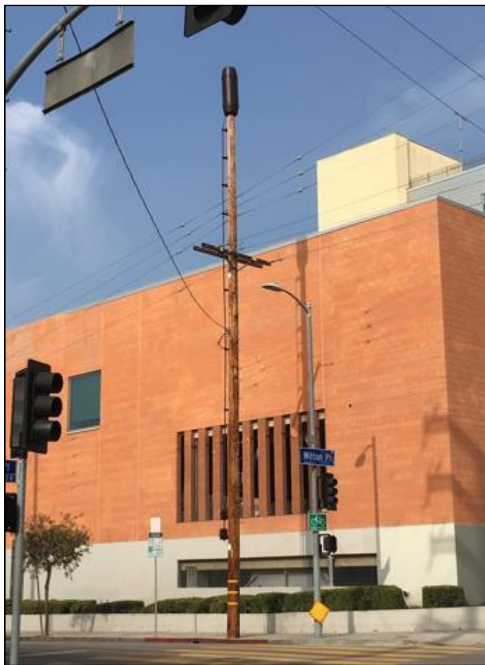
Figure 2: Pole-top antenna on a wood utility pole with tapered shroud.
