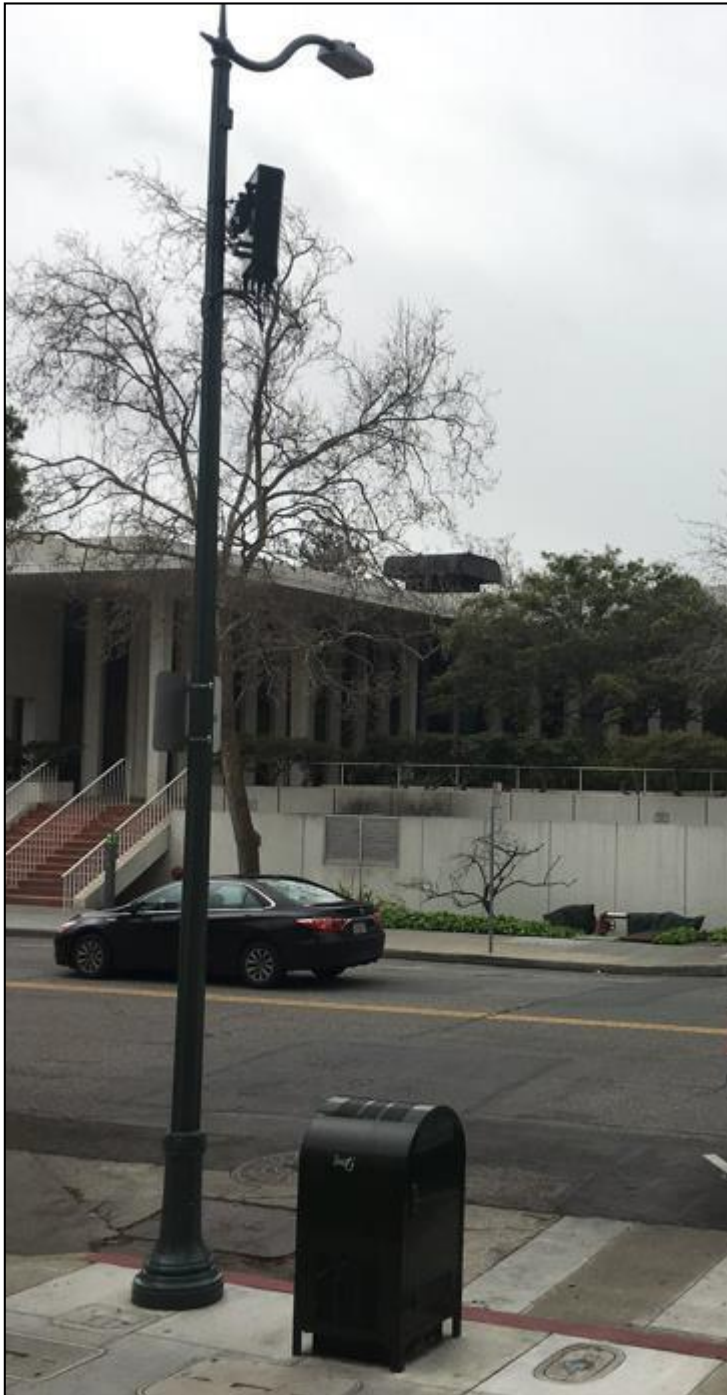
Figure 7: Ground-mounted accessory equipment concealed as a mailbox.
