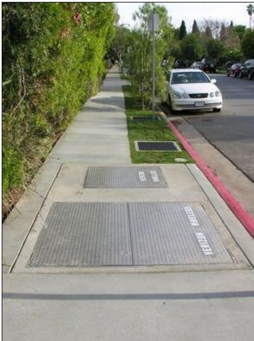
Figure 3: Flush-to-grade underground equipment vault.
